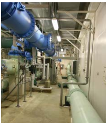
Typical piping runs at the Evansville Water Treatment Plant.
