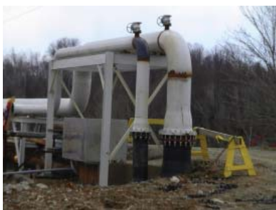
Example of piping at the AB Brown Power Plant.
